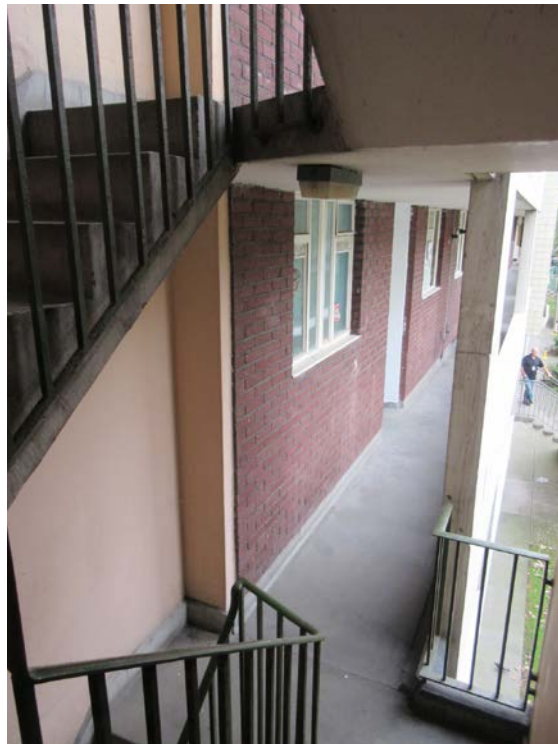
Close up detail of access decks and external tiled façade (top) and view of access deck from stair core (bottom).
